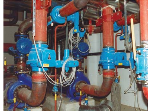
KHI ball valves in district heating system
