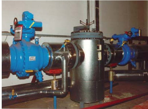
KHI ball valves in district heating system
