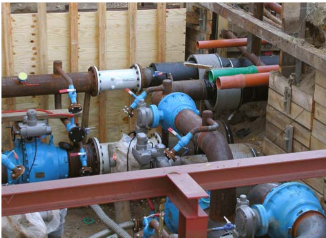
Installation site of Stadtwerke Kiel (Kiel's municipal utility): Klinger Ballostar KHSVI and Monoball ball valves
